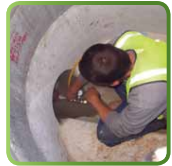
Typical ASTM F1417 Air Test
